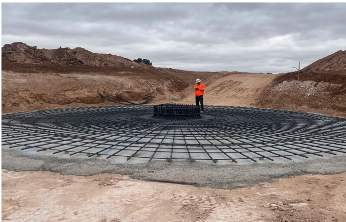
SunZia Wind Project
